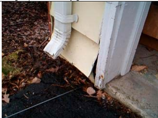
Example of downspout discharging adjacent to house
