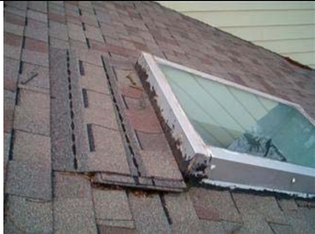
Shingles piled above skylight
