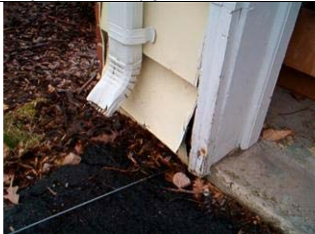
Example of downspout discharging adjacent to house
