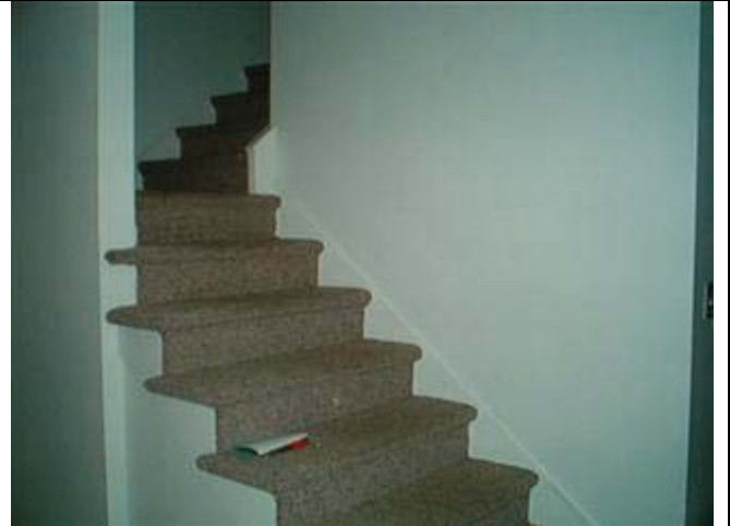
Example of missing rails and an open side at stairs
