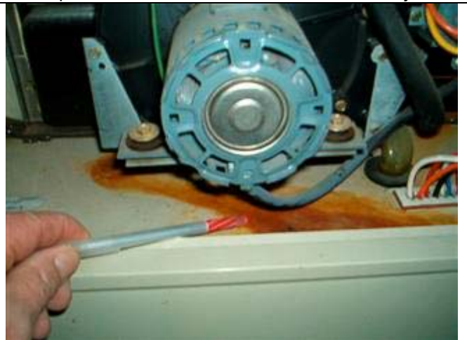
Corrosion in furnace cabinet
