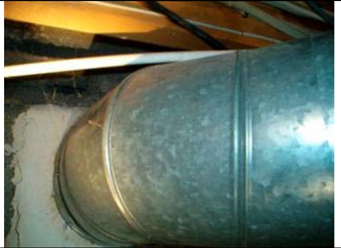
Inadequate clearance from water heater vent to joists
