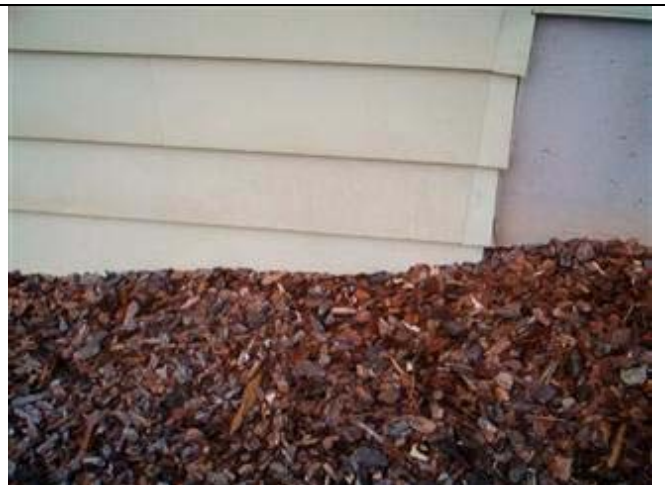
Example of soil/siding contact
