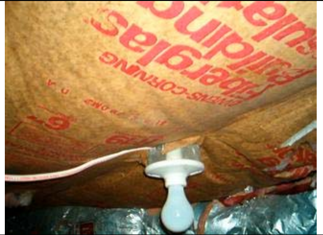
Insulation upside down in crawlspace with paper exposed
