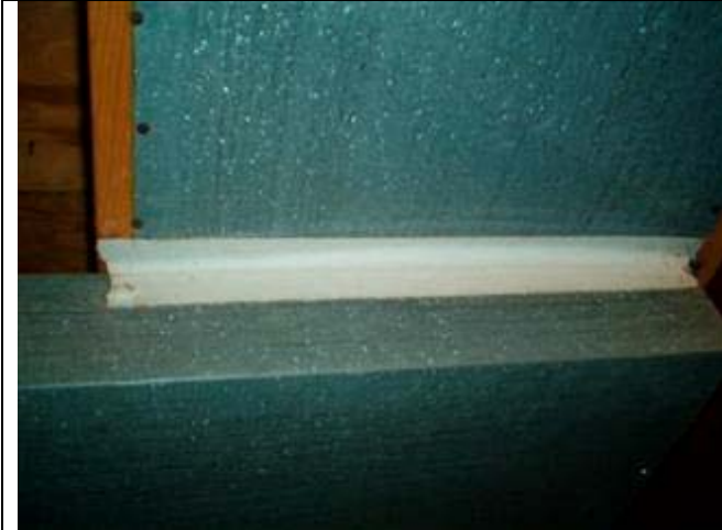
Suspected asbestos duct tape in basement
