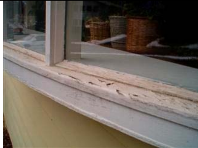
Example of peeling exterior paint
