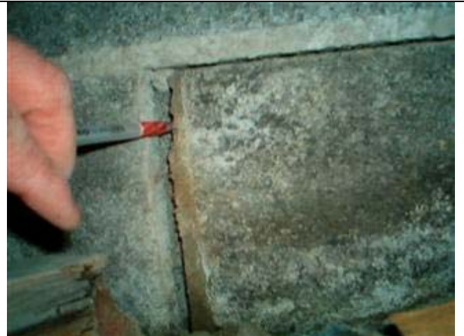
Crack and offset in crawlspace foundation
