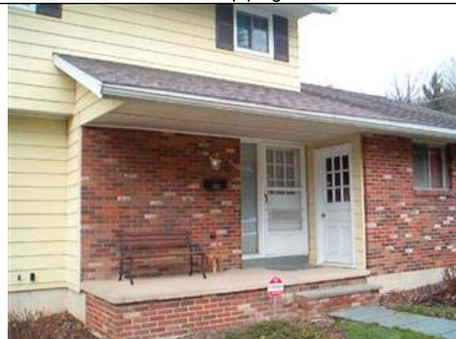
Missing corner post at porch roof, missing rails, excessive rise at step
