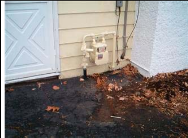
Gas meter unprotected at driveway
