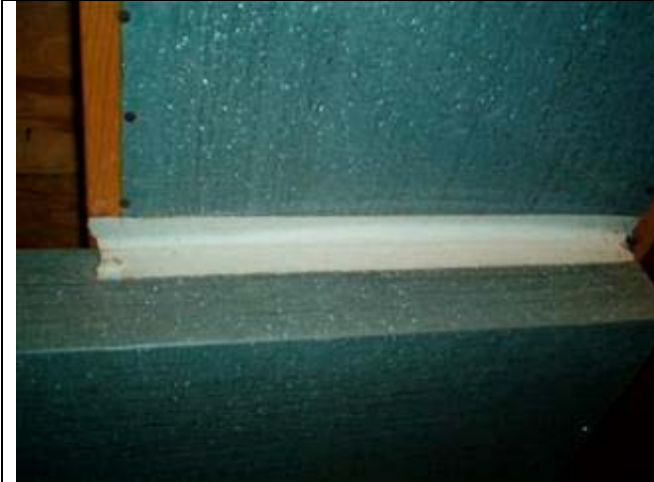
Suspected asbestos duct tape in basement
