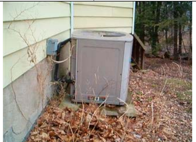
Air conditioner unit out of level
