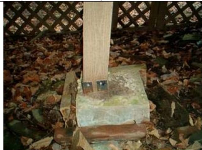
Settled footer, post out of plumb under deck
