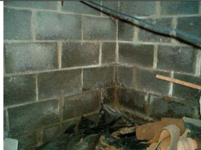
Damp conditions in crawlspace
