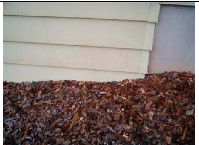
Example of soil/siding contact
