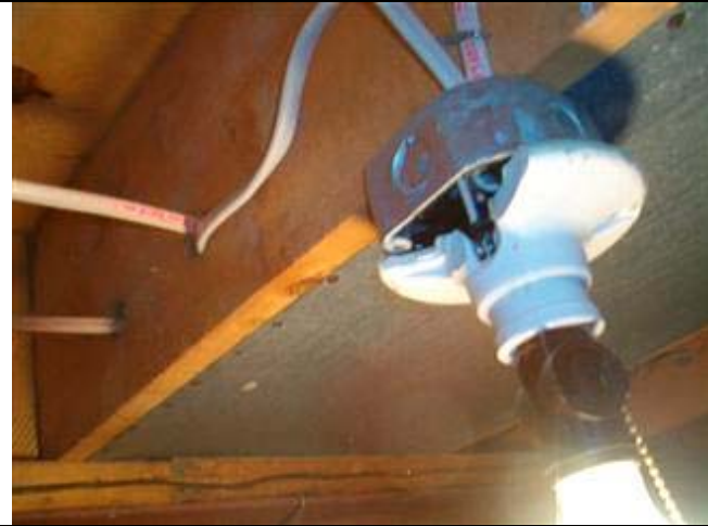
Broken light fixture above basement workbench
