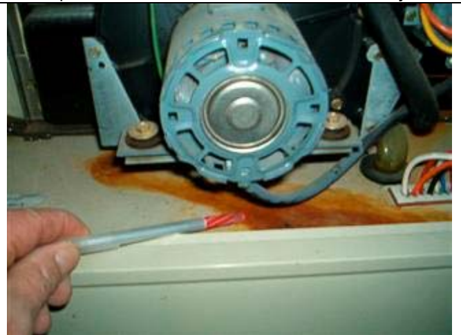
Corrosion in furnace cabinet
